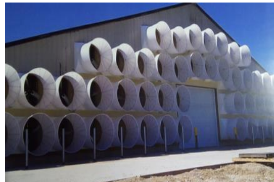
Figure 3: A typical ventilation
