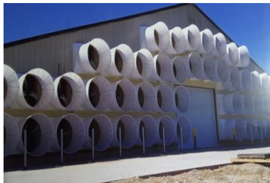
Figure 3: A typical ventilation
